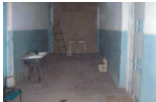
An example of the repairs needed at the Tsintskaro health post.
